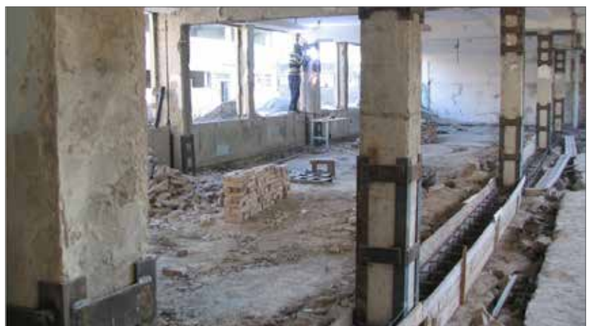
Figure 1. Following structural assessment of schools, the MPE rehabilitated 3,608 schools using a variety of retrofit techniques; another 2,470 schools underwent capital reconstruction, a form of intervention that included a combination of new construction and retrofit. Photo credit: Bakhtiar Nurtaev
